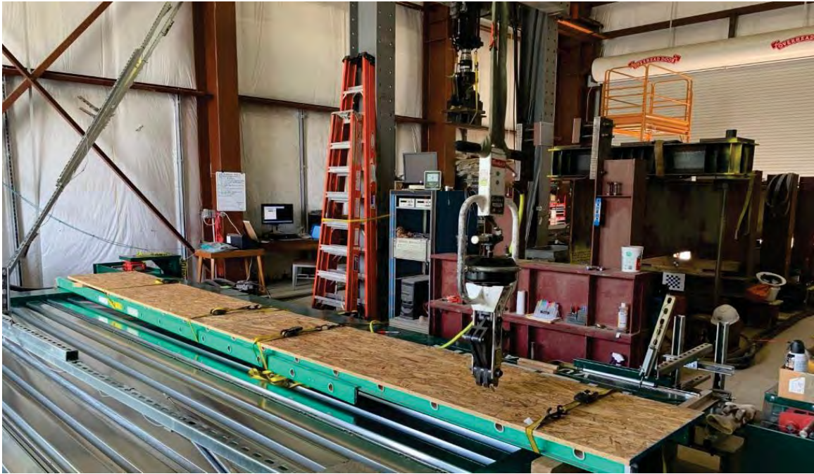
Figure 14: Construction platform for sidelap connections. The Punchlok – II tool was supported by the crane during specimen fabrication
