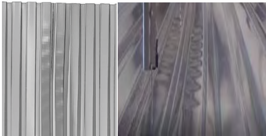
Local buckling near deck ends
